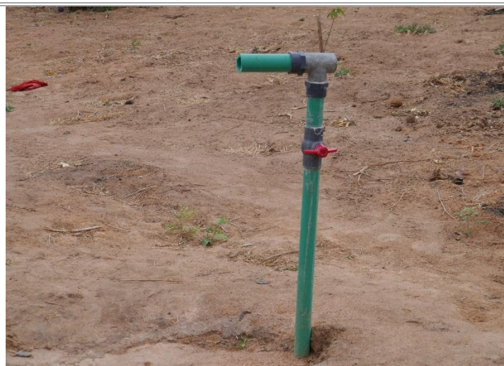
Parts of the water supply system at MAMOCOSO, funded by LIC
